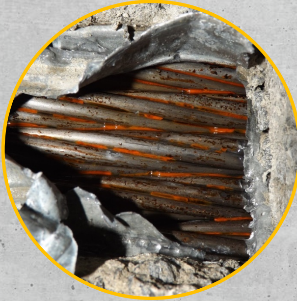
Grouting Defect Light Corrosion
