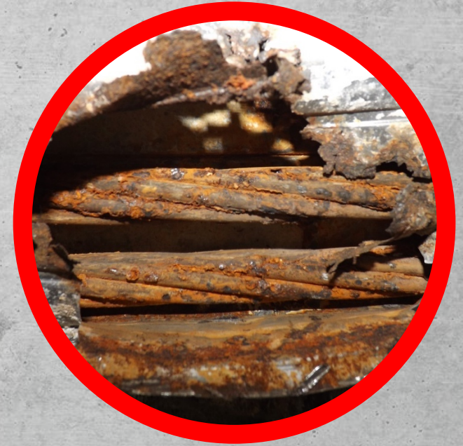
Grouting Defect Heavy Corrosion
